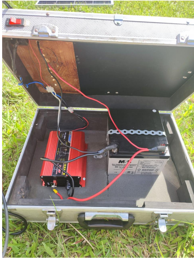
Figure 2: Inside the solar generator
